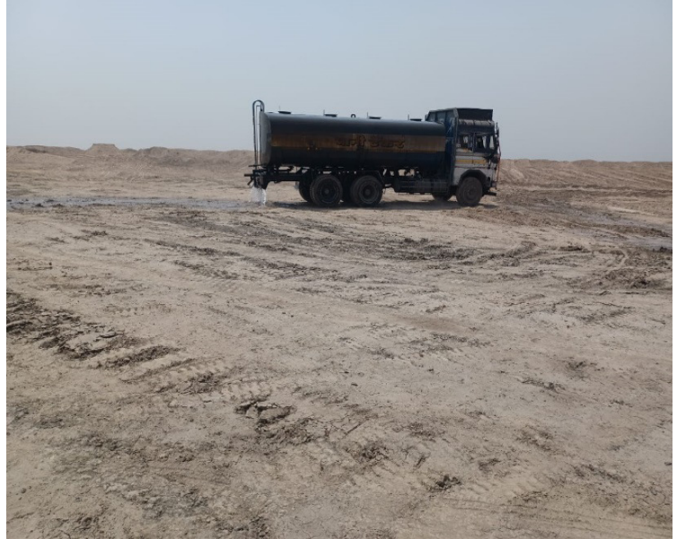
Figure 6 Truck mounted water tanker for dust suppression at fly ash back filling site
