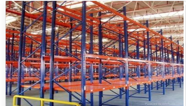
HRPO Grade in Racking System
